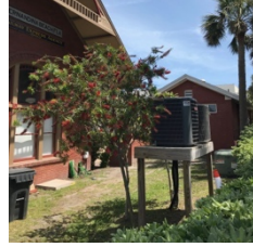
Figure 60. Other: Mitigation Strategy, Raised HVAC (Fernandina Depot)
