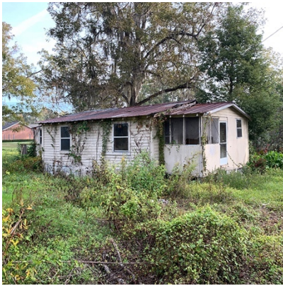
Figure 46. Poor => Unstable (a): Florida Cracker cabin, Monticello
