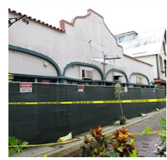
Figure 63. Other – Structural Failure, Aviles Street, St. Augustine
