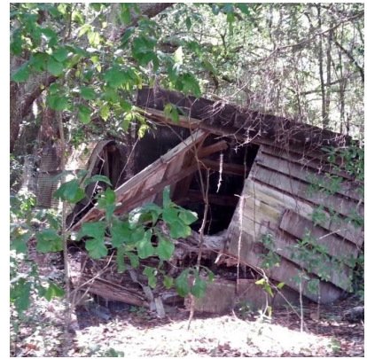
Figure 48. Poor => Unstable (c) Manning Turpentine Shack
