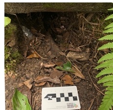
Figure 55. Animal Disturbance, Gopher Tortoise Tunneling Under Foundation – Monticello
